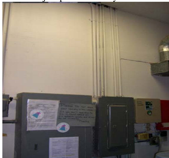
Sign in laundry room telling staff not to leave laundry in washer due to the smell in the room
