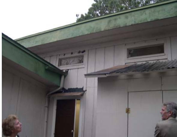
Viewing the dry rot
